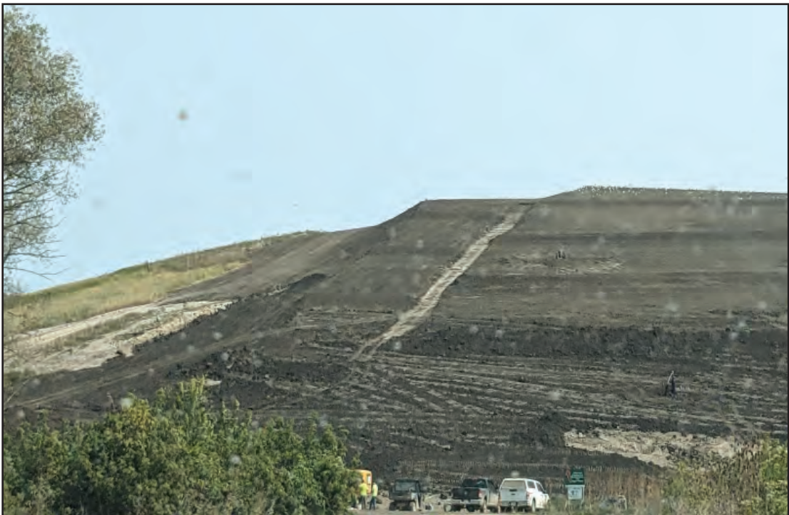
Top soil placement on new cap nearly complete; armoring for downslope flume
